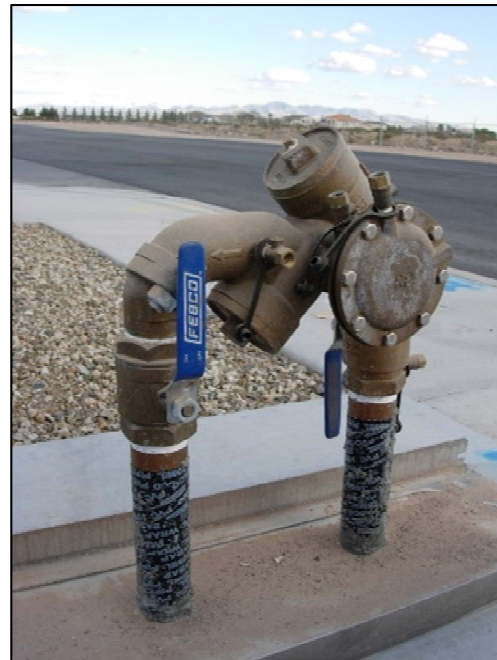
Image: Commercial Backflow Assembly
