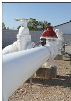
Image: LVVWD Groundwater Well
