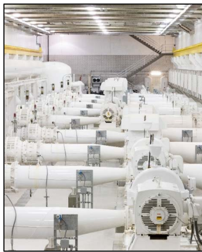
Image: LVVWD Pumping Station
