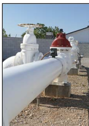
Image: LVVWD Groundwater Well
