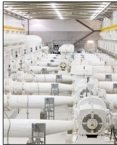
Image: LVVWD Pumping Station
