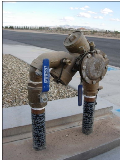
Image: Commercial Backflow Assembly
