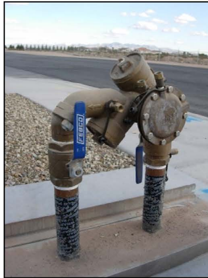
Image: Commercial Backflow Assembly
