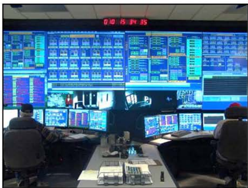
Image: Supervisory Control and Data Acquisition (SCADA) center.
